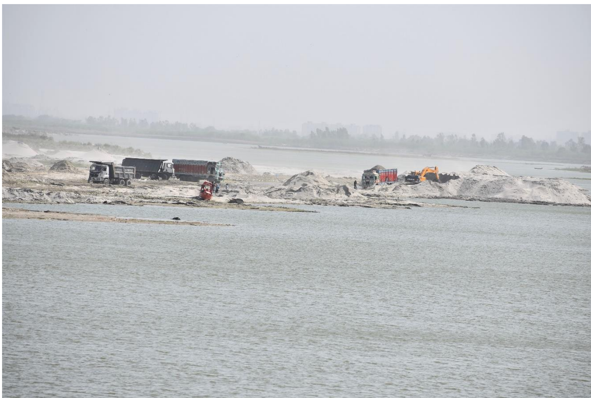
Image 34 : Sand Mining From Ganga River Near Between Bithoor In Kanpur Nagar Distt. And Pariyar In Unnao Distt.
