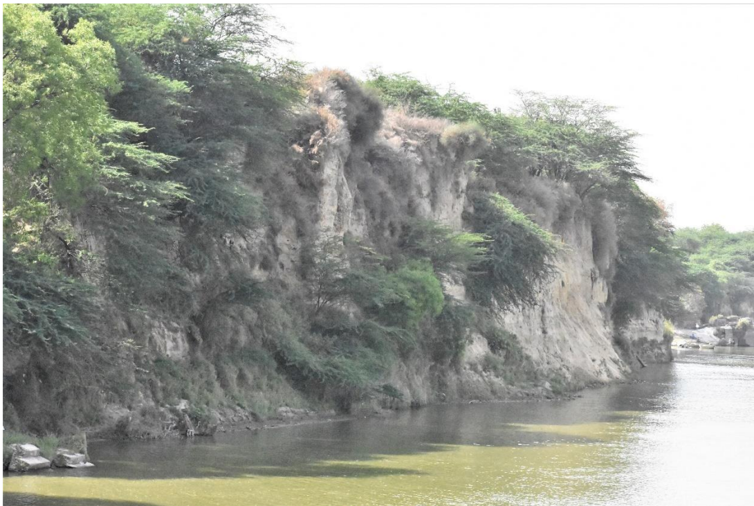
Image 33 : Erosion Impacts On Dhruv Teela Near Bithoor
