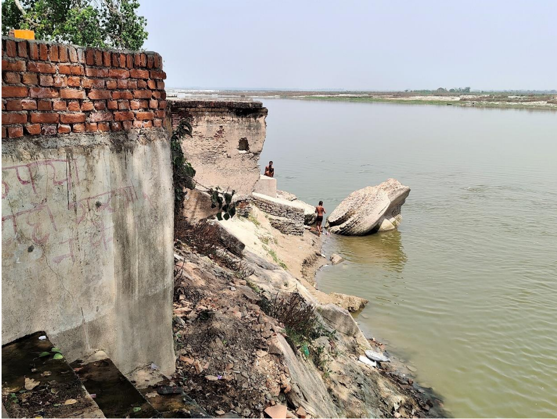
Image 32 : Damage Caused By Bank Erosion Near Najabgarh Ghat In Kanpur Nagar Distt.
